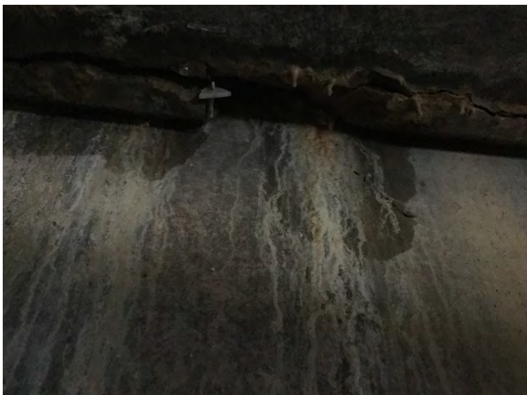
Damage to panel 1 right bank
