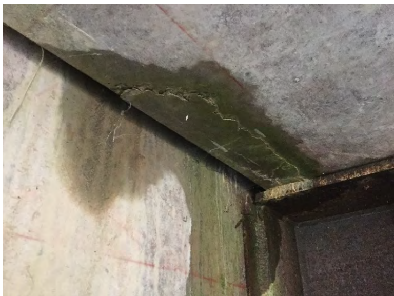
Damage to panel 1 at right bank
