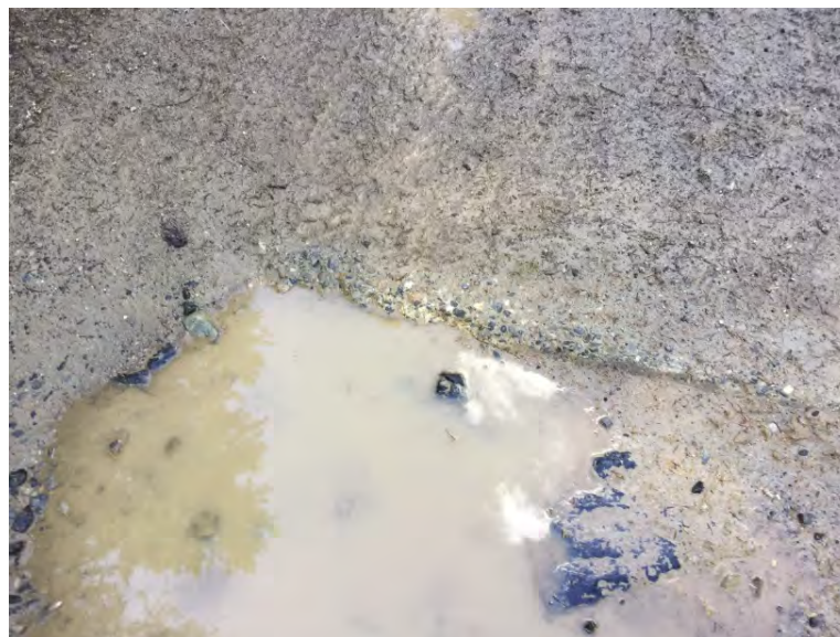
Damage noted to top of right bank ballast wall
